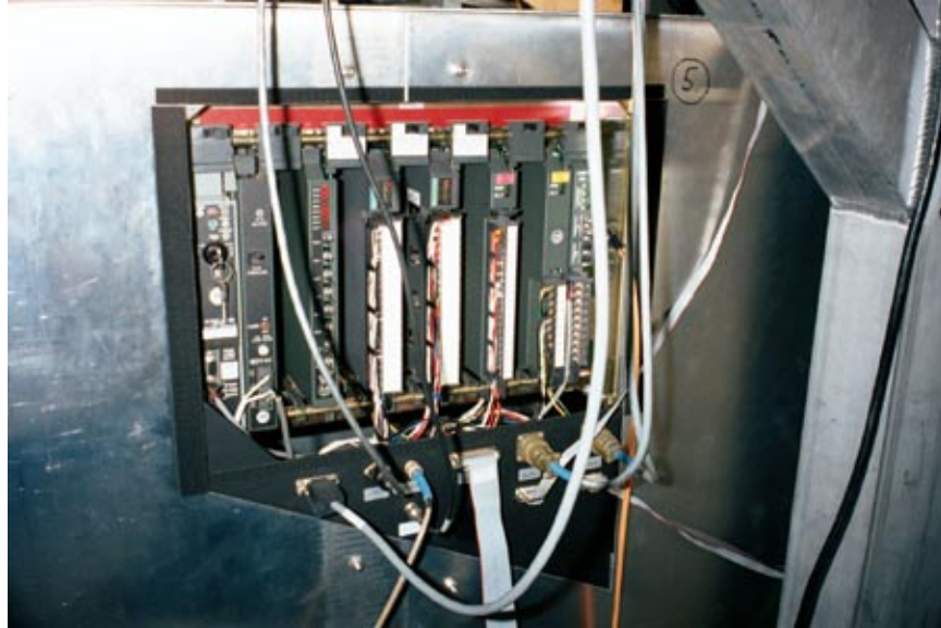
Figure 2-25: The programmable logic controller used to remotely control the PCI system.
