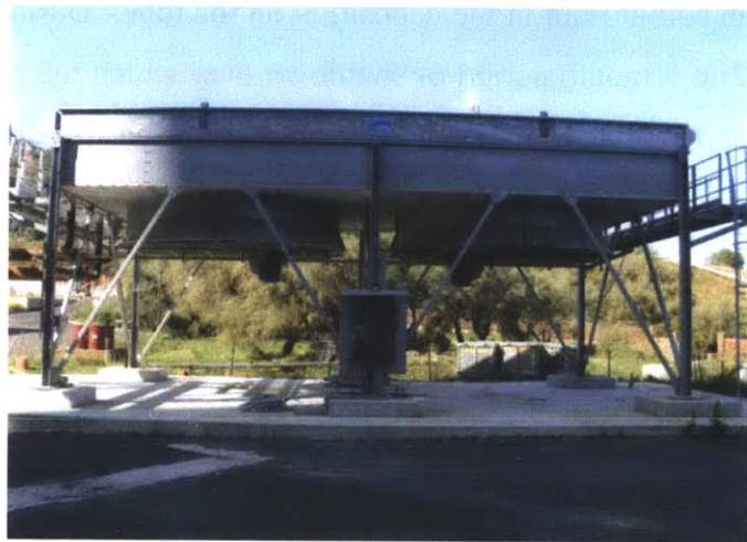
Figure 5-Picture of the dry cooling tower at the Larderello Power Plant (courtesy of ENEL).
