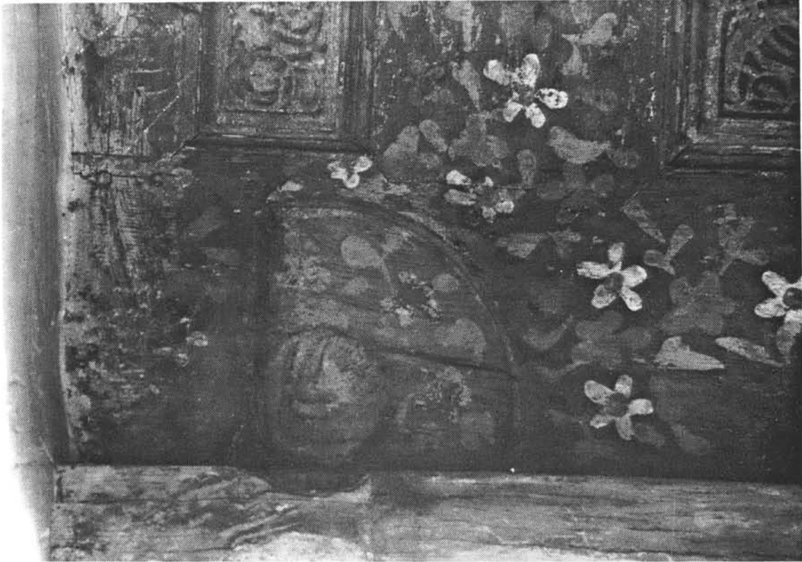
Figure C5.6g: Qā'a of Aḥmad Bey Kohya. Detail of soffit of the majlis showing recess for door hinge.
