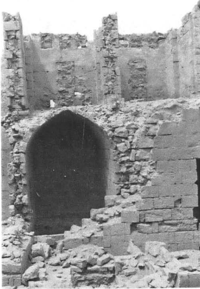
Figure A1.12g: Complex of Īnāl. Remains of two apartments, showing vaulted ground floor.
