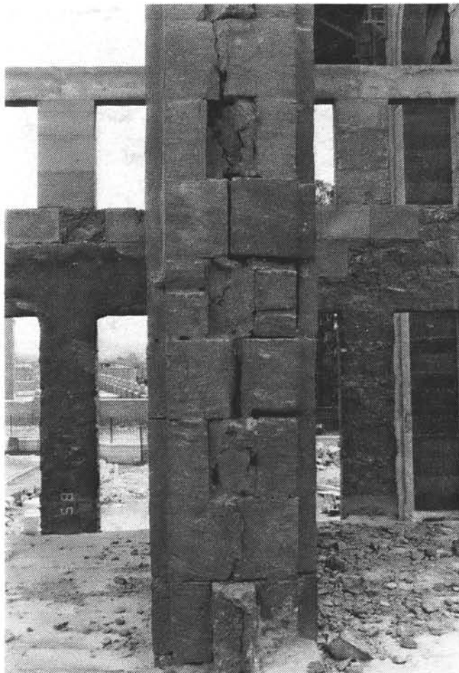
Figure A1.7d: Complex of Qurqumās. Construction of party wall between apartments in khanqā .
