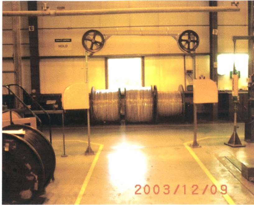
Figure 7-4 CV Line Personnel Pass-Through
