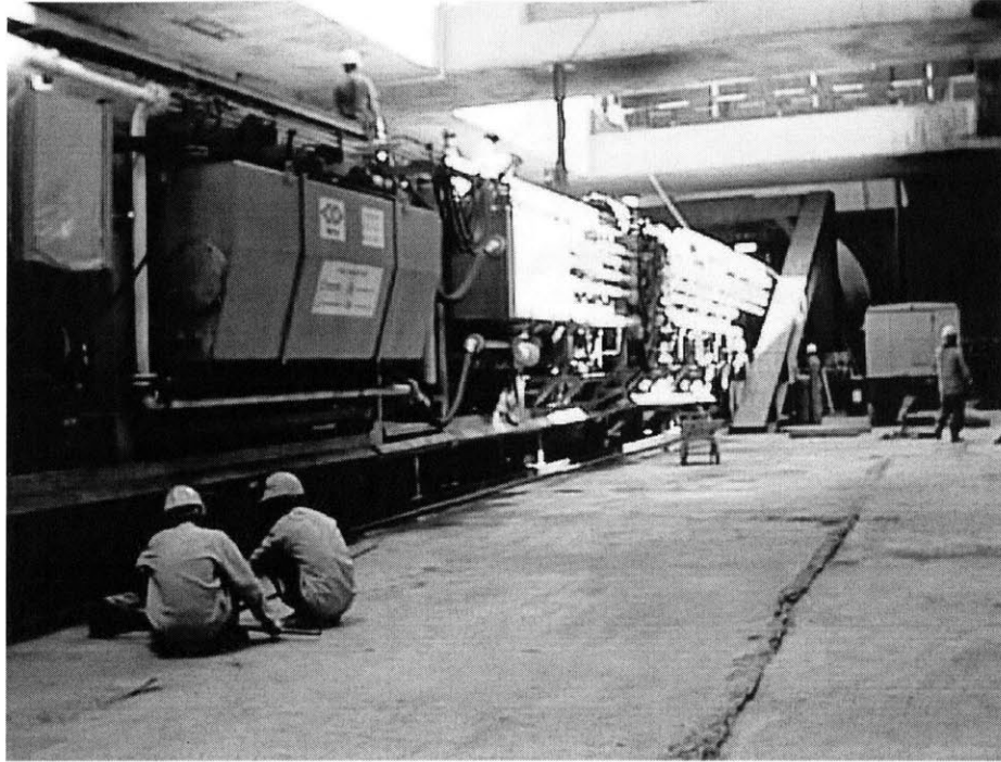
Figure 5.42 Backup equipment installed behind the SB shield inside Sirikit station
