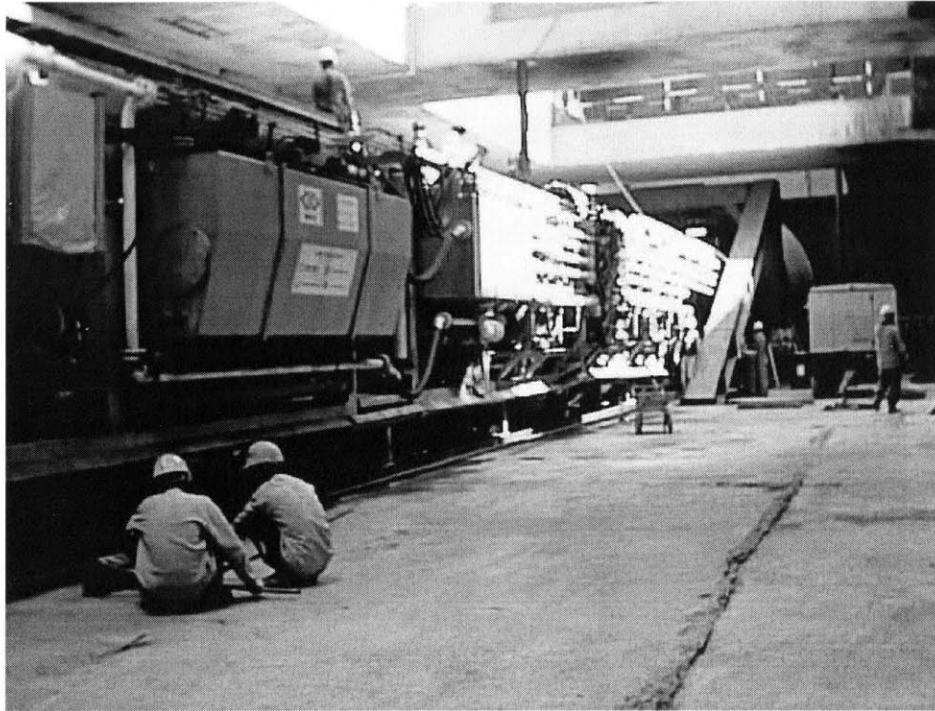
Figure 7.10 Back-up equipment train (Sirikit station)
