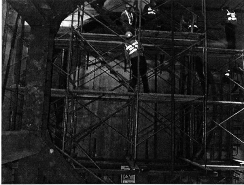
Figure 5.18 Diaphragm wall prepared for shield cutting through in Ratchada station (North Tunnel Section)
