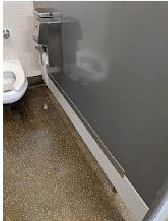
Figure 4.10: Toilet fixture in enclosed stall with additional privacy panels (the white strip).
