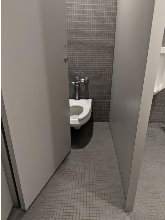
Figure 4.11: Fully enclosed restroom stall with toilet fixture.
