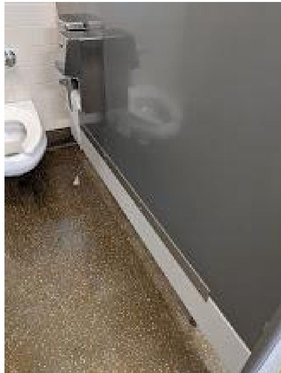
Figure 7.4: Toilet fixture in enclosed stall with additional privacy panels (the white strip).
