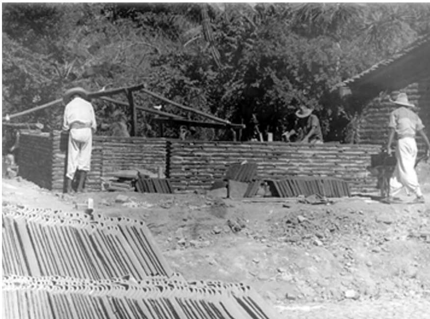
Men building a house near Mexico City, ca. 1940. Hombres Construyendo Casa , Ca 1940, 12.7 x 17.8 cms, Ca 1940, Fototeca Nacional, https://mediateca.inah.gob.mx/islandora_74/islandora/object/fotografia%3A399247 .
