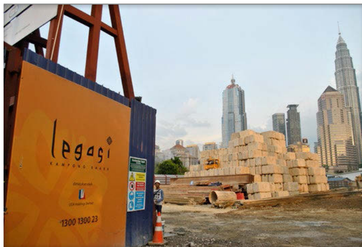
Figure 9. The Legasi condominium project occurs on the site of Kampung Bharu's former Sunday night market. Photo credit: April Ognibene, 2016
