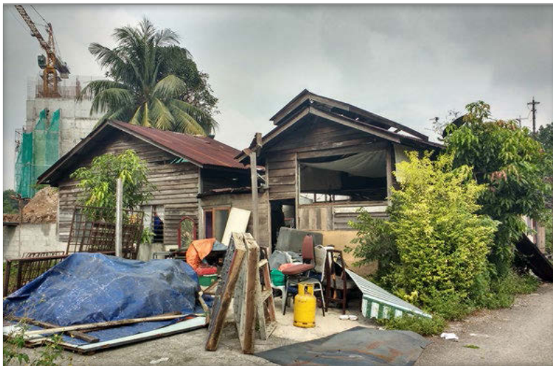
Figure 13. A house in Kampung Chubadak Tambahan designated for demolition for the private housing project. Photo Credit: Vishnu Prasad, 2016
