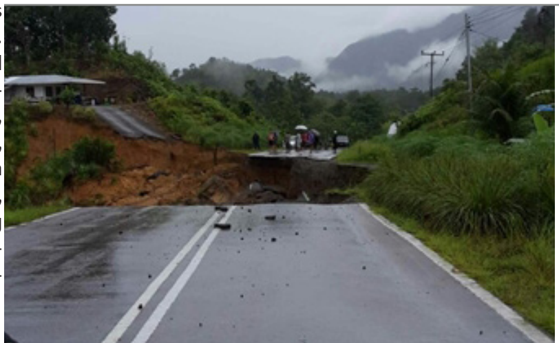
Figure 22. Road off of Jalan Puncak Borneo (near Bengoh Dam) caved in after heavy rains. © Borneo Post. All rights reserved. This content is excluded from our Creative Commons license. For more information, see http://ocw.mit.edu/help/faq-fair-use/
