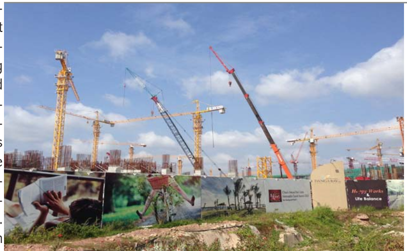
Figure 4. Construction underway in Danga Bay, one of several large Chinese-funded residential real estate developments on reclaimed land in Johor Baharu. Photo by Andrew Binet, 2015.
